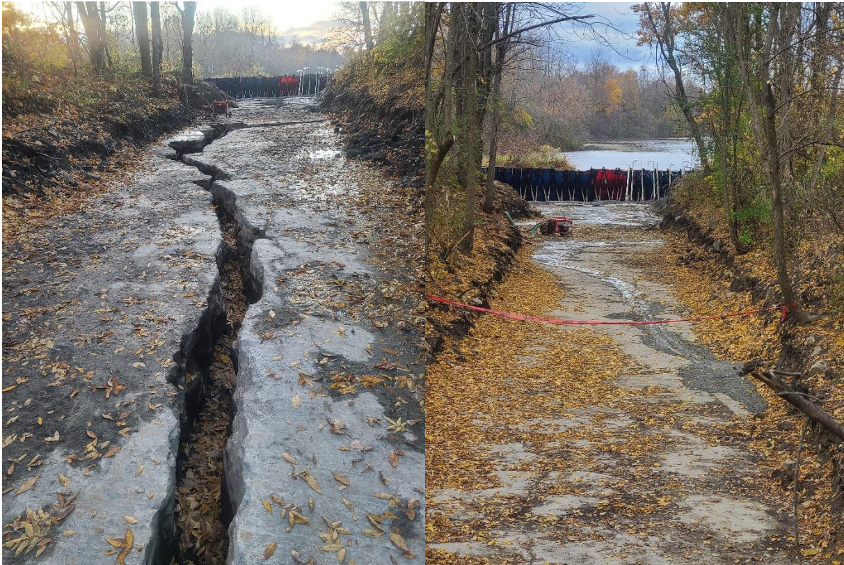
Figure 8. Fissures in Mill Race side channel before (left) and after filling with cement (right) at Frog Farm Dam in NY.
