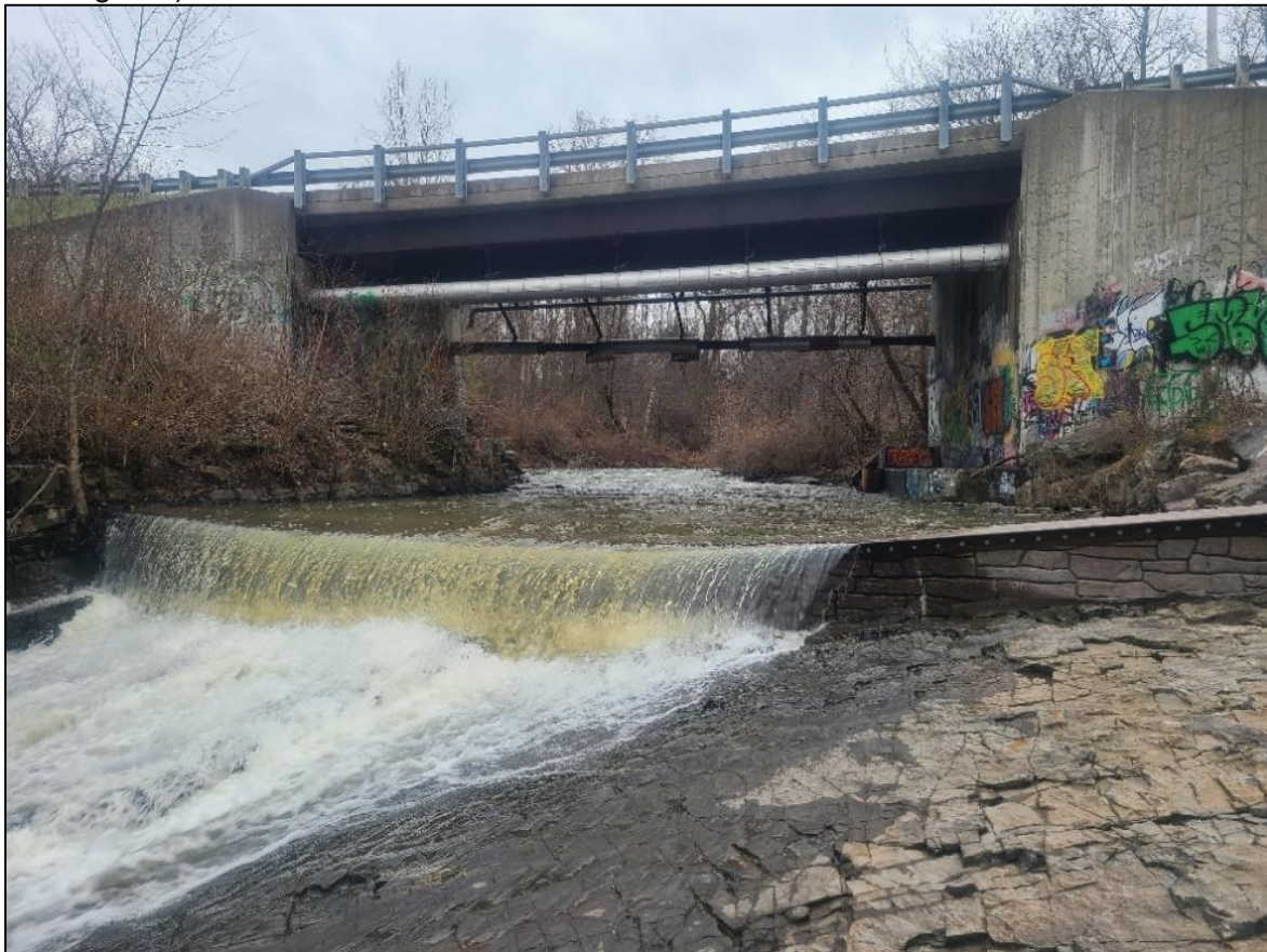
Figure 7. New low-head barrier on the LaPlatte River at Shelburne Falls in Vermont.
