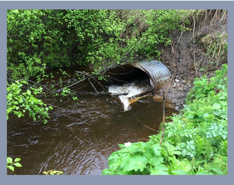
An undersized culvert in the Tyonek Creek watershed that is typically plugged with debris. Credit: USFWS
