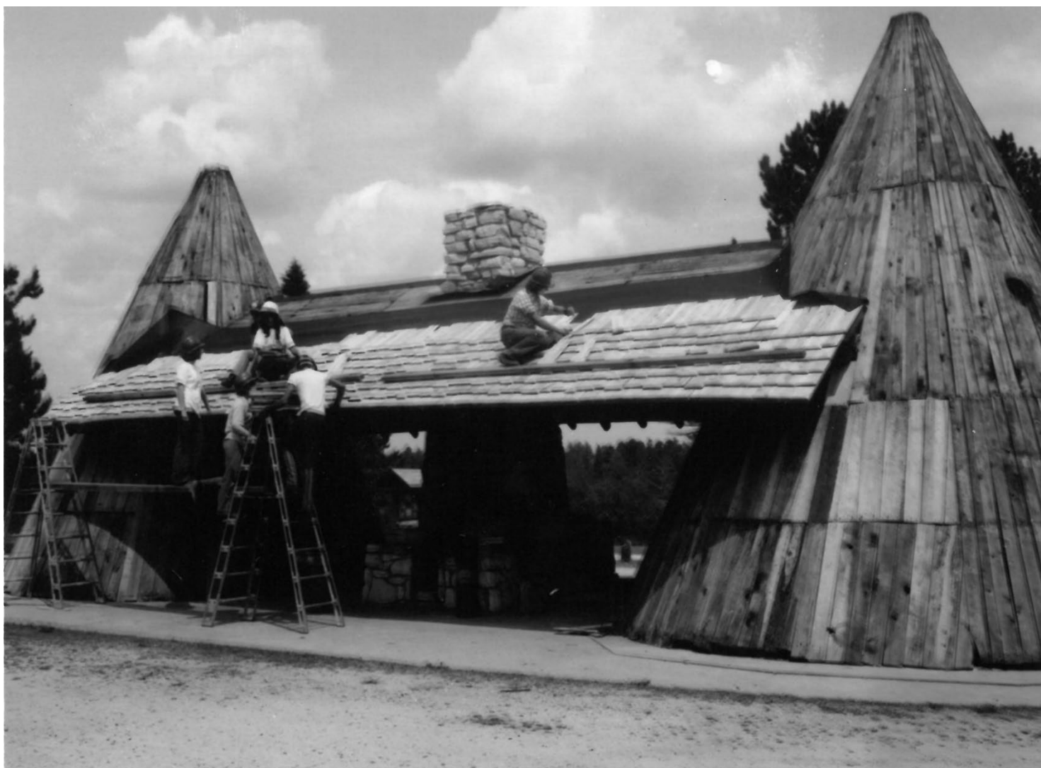
Photo 5: The Show Pool Shelter in 1974 when it was being covered with cedar shakes for the first time.
