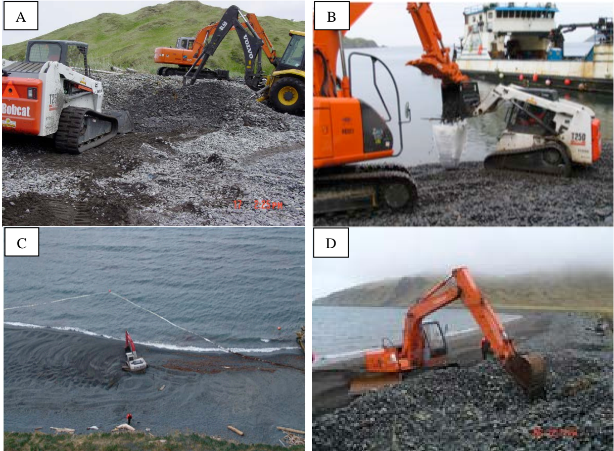
FIGURE 3.1 EXAMPLES OF CLEANUP ACTIVITIES USING EXCAVATING MACHINERY A. Dry tilling to expose buried oil (2 June 2005). B. Excavation of oiled sediments (4 July 2005). C. Berm relocation test (27 May 2005). D. Dry tilling (15 June 2006).
