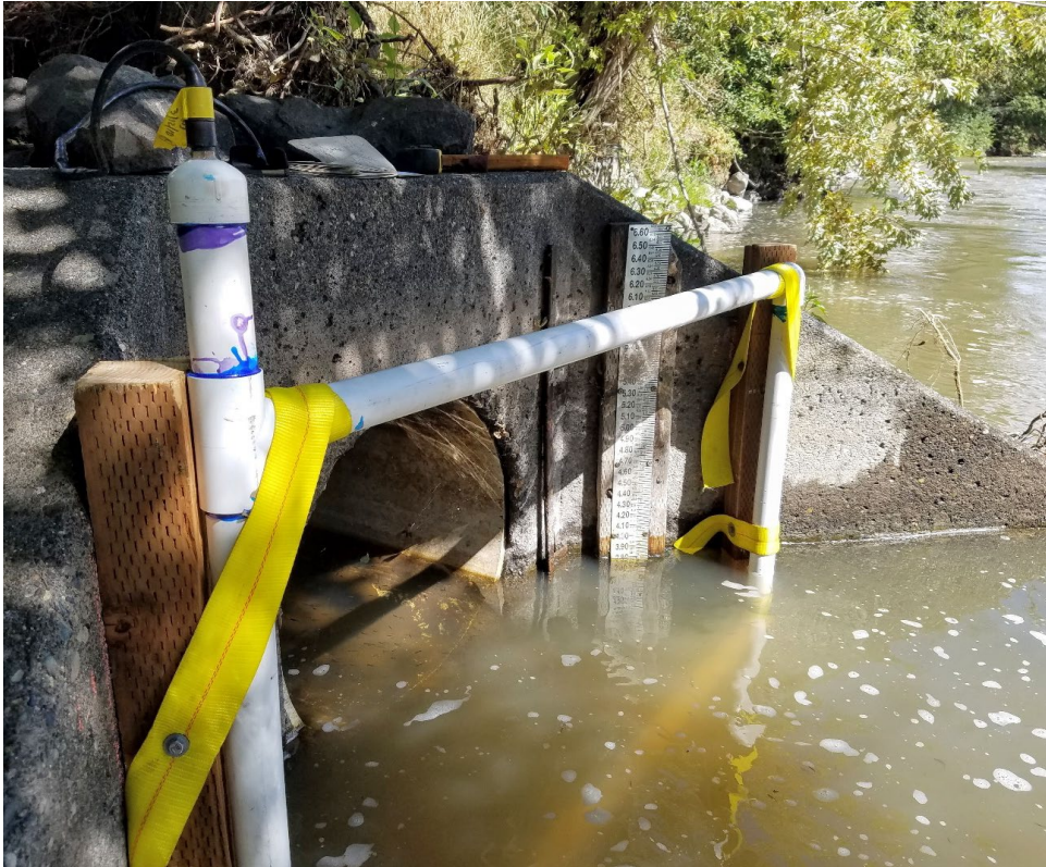
Figure 4. Fixed PIT antenna at the bypass outfall of the Feed Diversion Canal.
