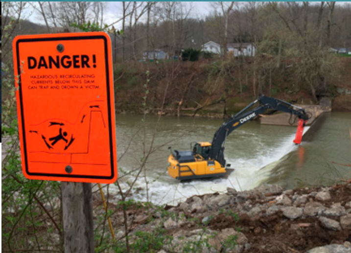
(Top) Removal of the Highland Dam on the West Fork River in West Virginia.
