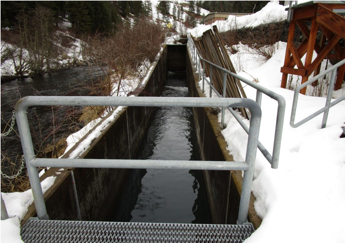
Figure 4. Lower ladder at the LH, in operation since 2018 in conjunction with the upper ladder and weir.
