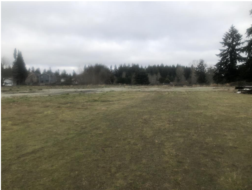
Photo 8. View north from PP4 of gravel parking area and building demolition site (January 21, 2021).
