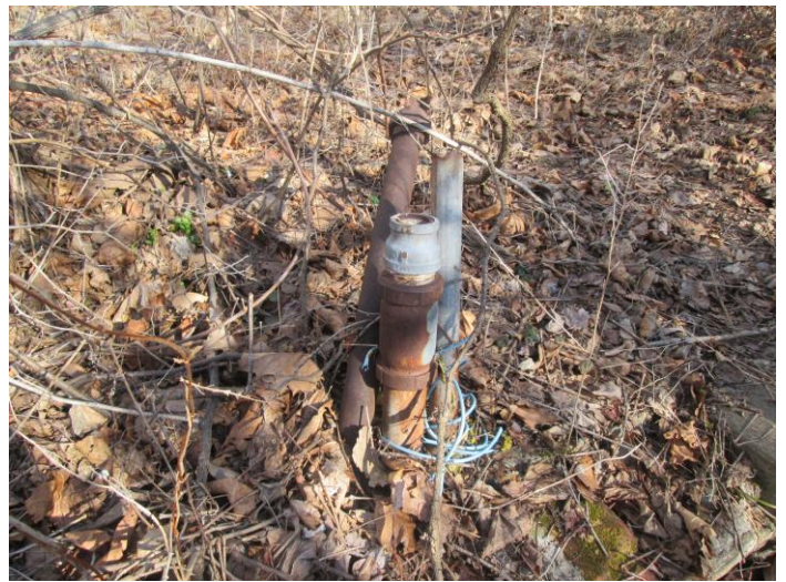
Photo 16 - Unknown subsurface piping
