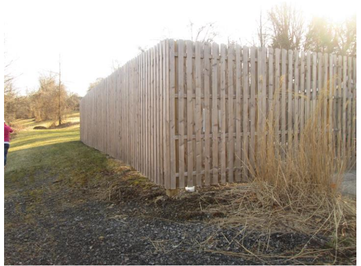
Photo 2 - Sewage pumping station
