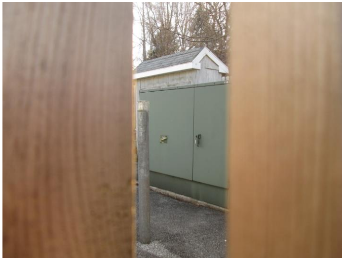
Photo 3 - Transformer within sewage pumping station
