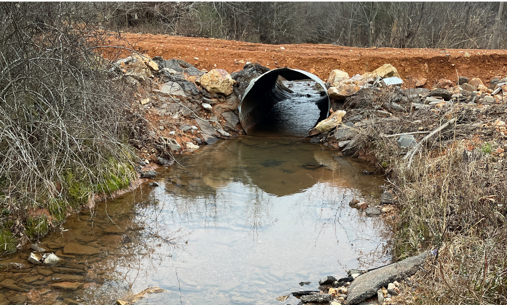
An undersized culvert in St. Clair County, Alabama, caused flooding issues for the local community. Photo credit: USFWS
