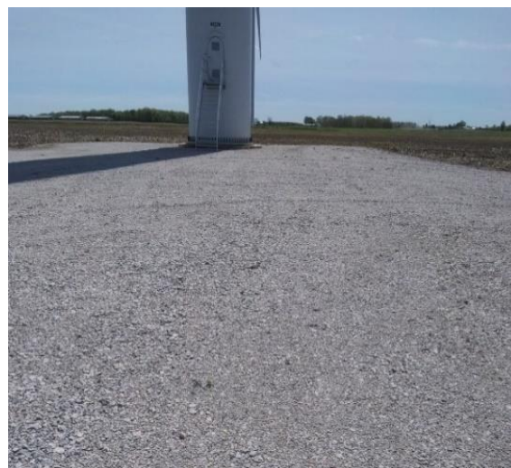
Figure 2. Representative photo of conditions in a 100-meter road and pad plot at the Hog Creek Wind Farm, Hardin County, Ohio.
