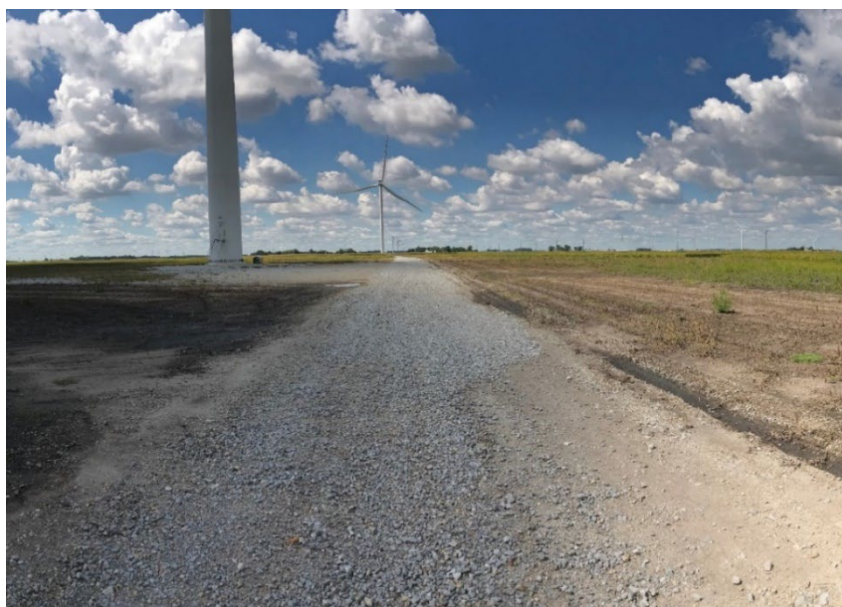
Figure 3. Representative photo of conditions of a 100-meter road and pad plot at Indiana Crossroads Wind Farm, White County, Indiana.
