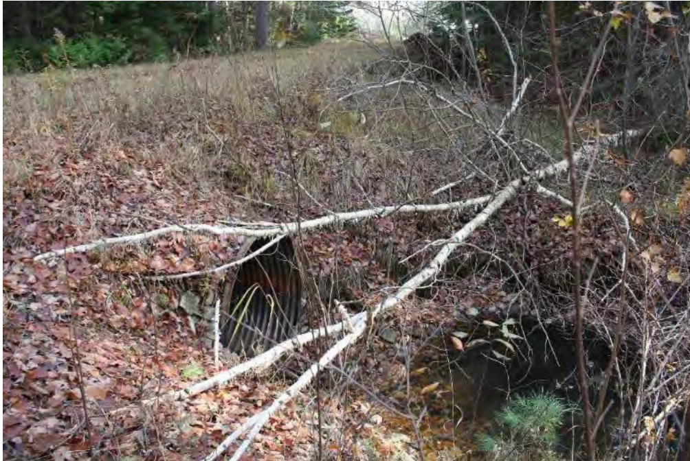
Figure 27 Project Area, Driggs River Road Delta Creek Culvert, view to the southeast
