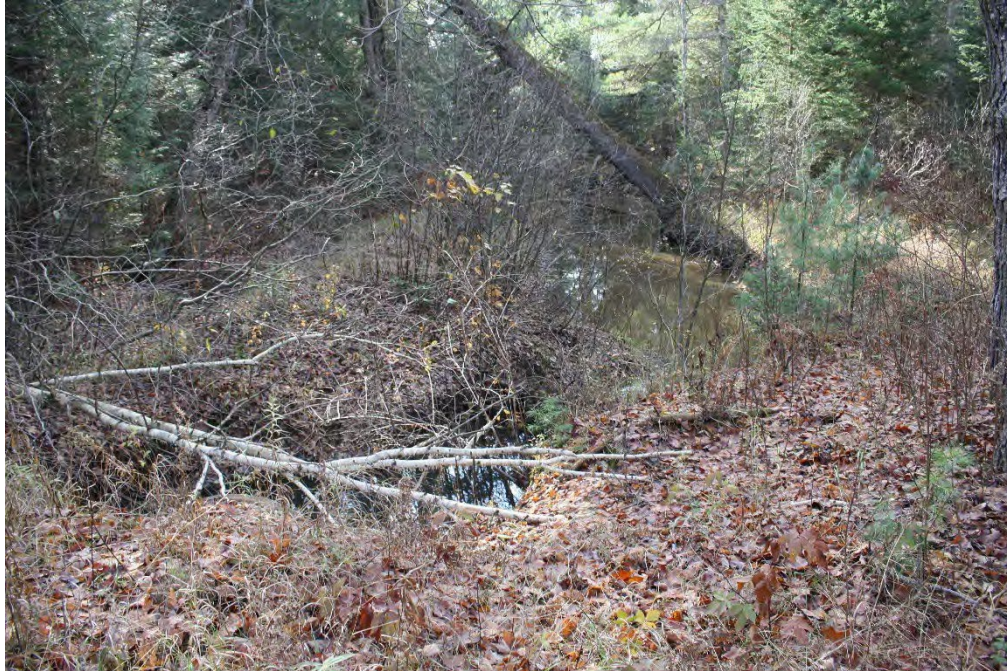
Figure 21 Project Area, Driggs River Road Delta Creek Culvert, view to the west
