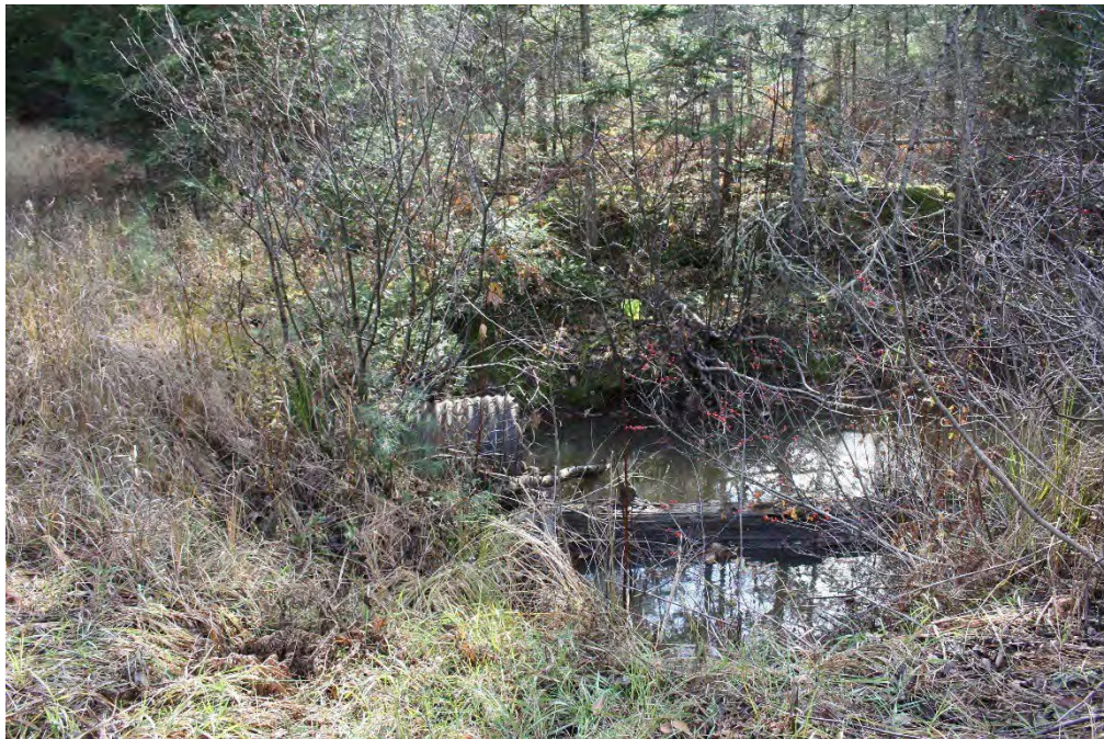
Figure 22 Project Area, Driggs River Road Delta Creek Culvert, view to the southeast
