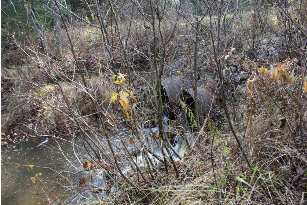
Figure 23 Project Area, Driggs River Road Delta Creek Culvert, view to the south
