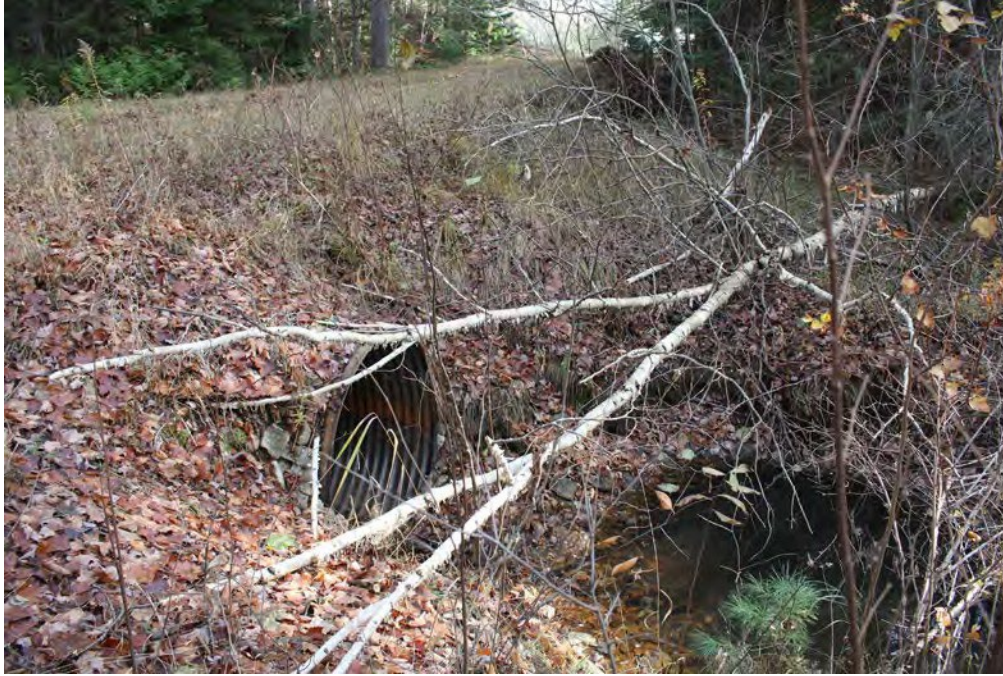
Figure 1. Route 405 Driggs River Road over Delta Creek Culvert (1), view to the south-southeast
