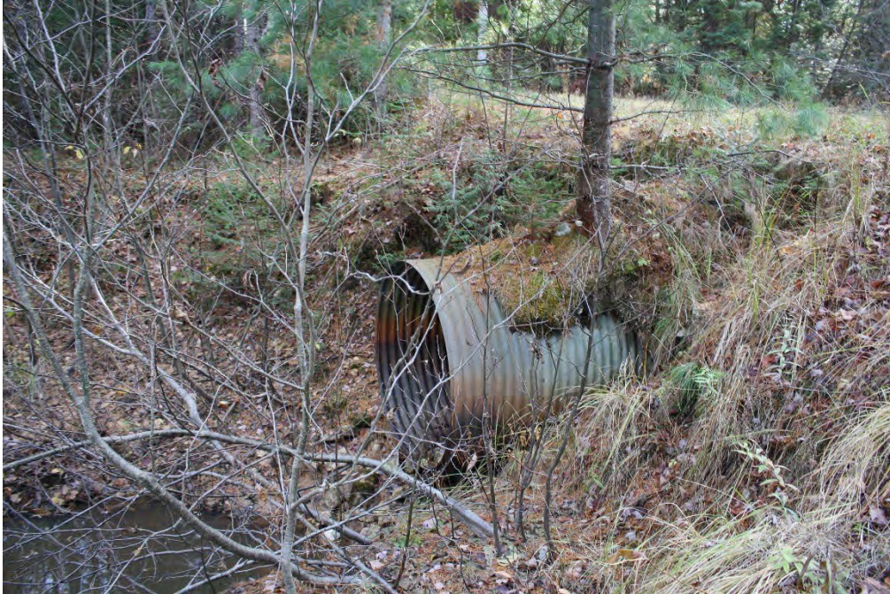
Figure 25 Project Area, Driggs River Road Delta Creek Culvert, view to the south
