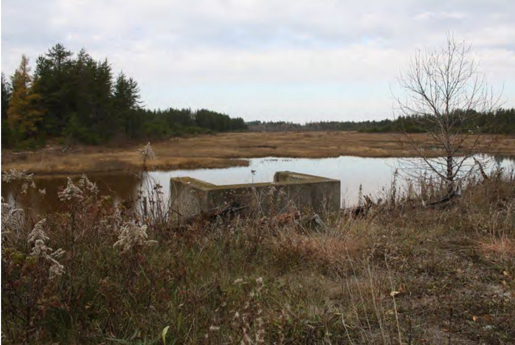
Figure 1. Delta Creek Pool to Delta Creek water control structure, view to the north
