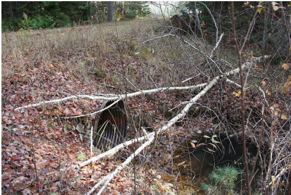
Figure 20 Project Area, Driggs River Road Delta Creek Culvert, view to the southeast
