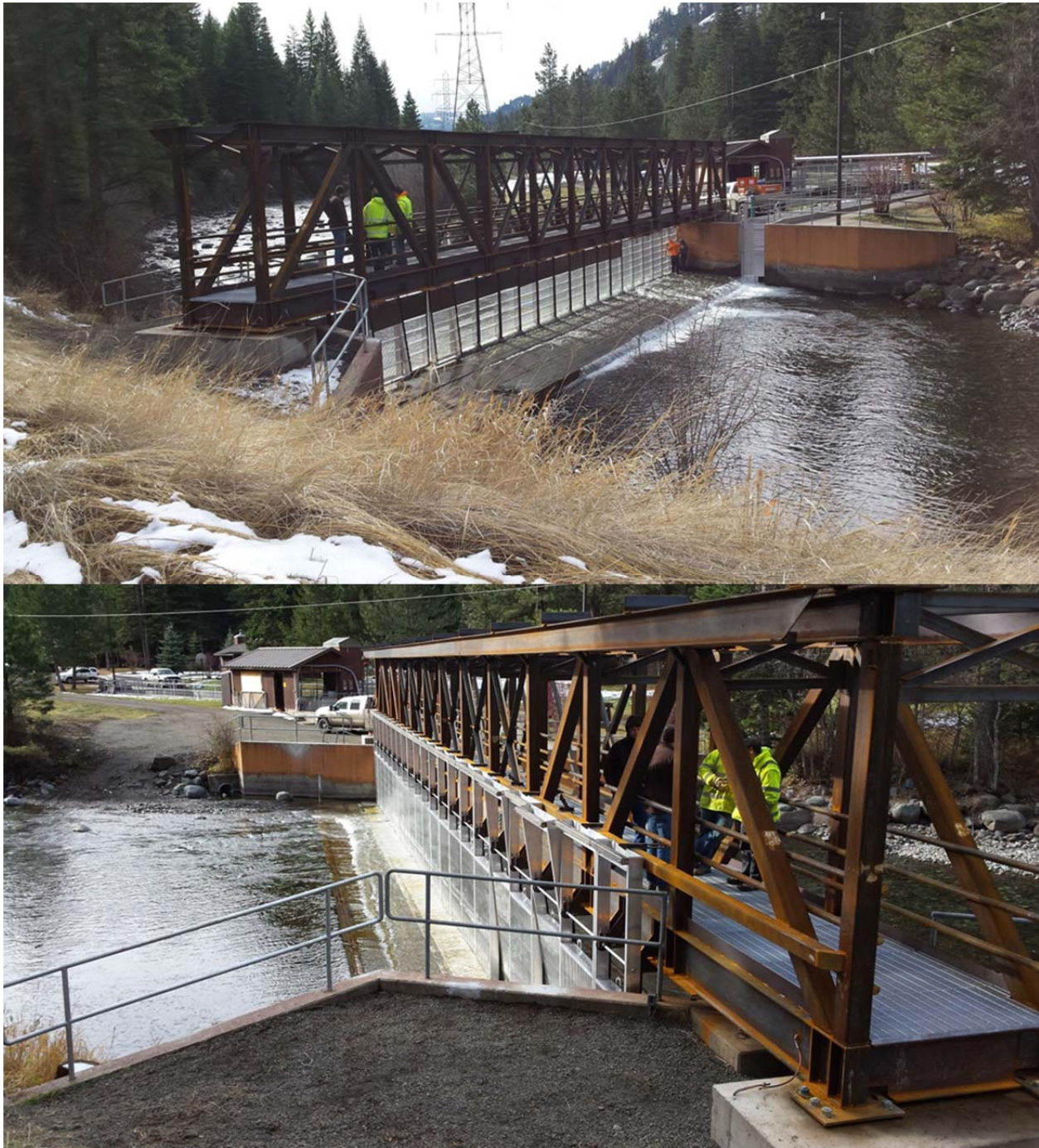
Figure 1. Pictures of the new bridge-style weir installed at the Imnaha River Acclimation Facility and Brood collection ponds during October 2015. Weir panels are in the “down” position and pivot from the lower portion of the bridge to operate. Photos by USFWS – Lower Snake River Compensation Plan Office.
