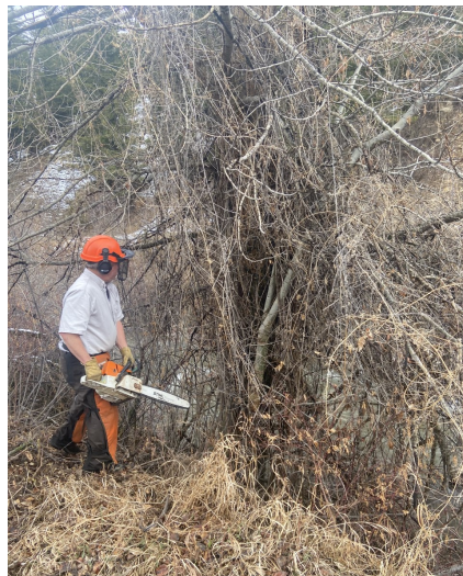
Directly behind the shop and above ground storage tanks.
