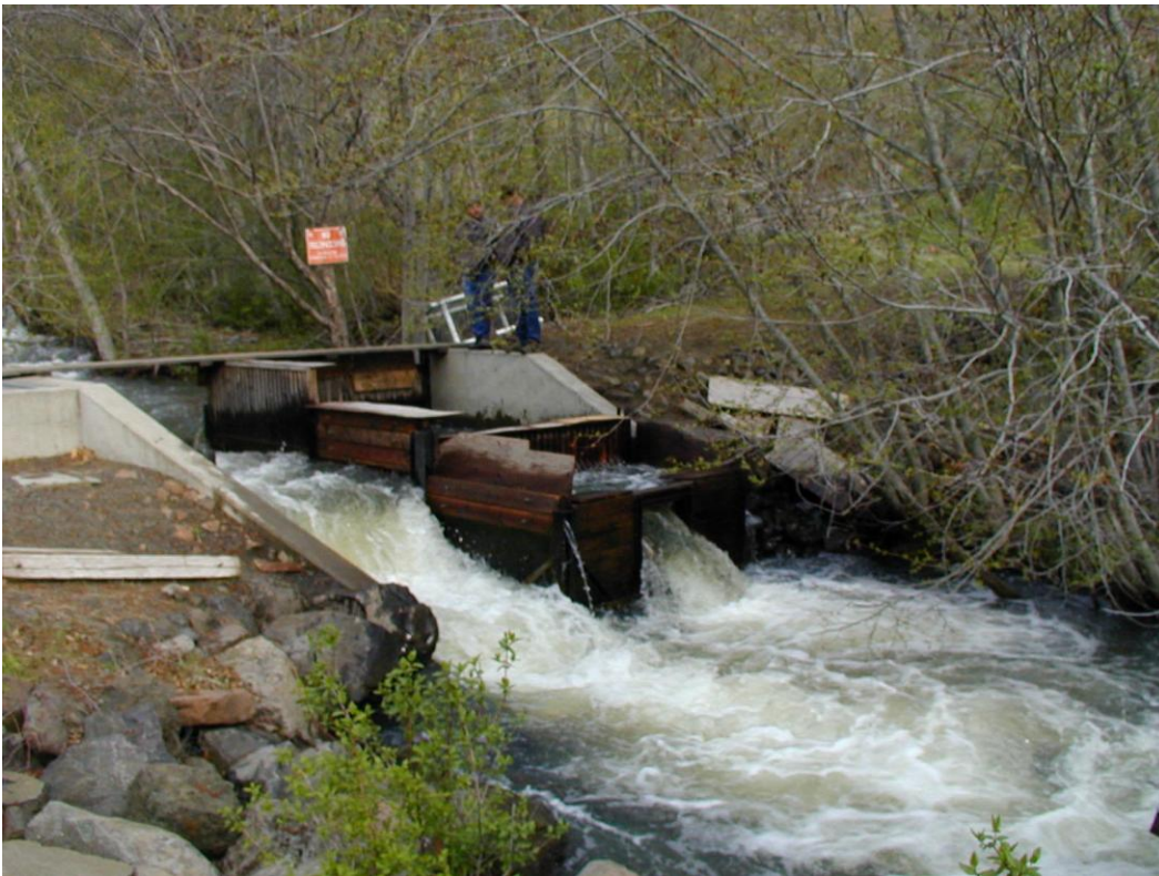
Photo 1. Cottonwood Adult Trap during high stream flows. Fish can bypass the trap in the left channel. The trapping area is located where is the spill is on the right channel.
