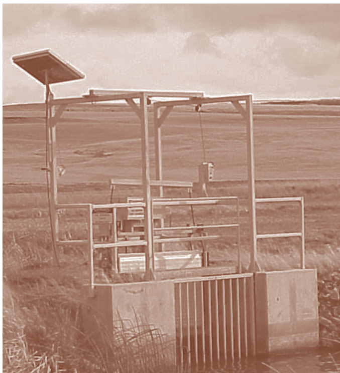
Bridge Creek Solar-powered Fish Screens, USFWS
