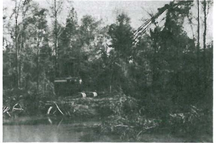
Figure 17. Dragline being used to remove compacted debris and sediment at major blockage (Condition Four).
