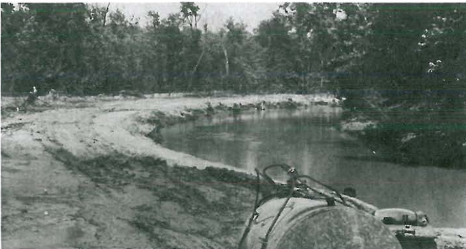
Figure 16. Debris and sediment removal was accomplished by working from one side of the stream. Selected trees were cleared to allow equipment access and operation. Trees have now grown back on the cleared side.
