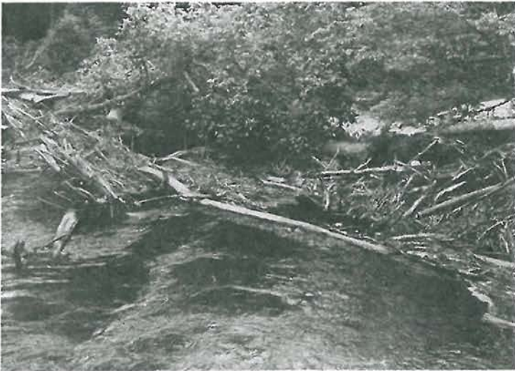
Figure 5. Log crossways of stream channel, trapping additional debris and restricting flow. Flow problems are likely to increase in the near future. Such accumulations may be removed.
