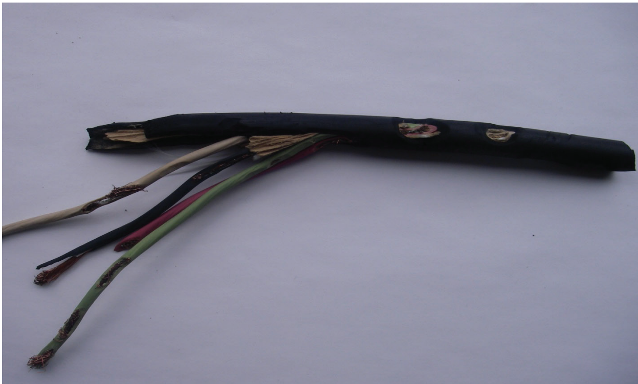
Figure 1. Damage inflicted on the lower spillway antenna by a suspected beaver in May, 2014
