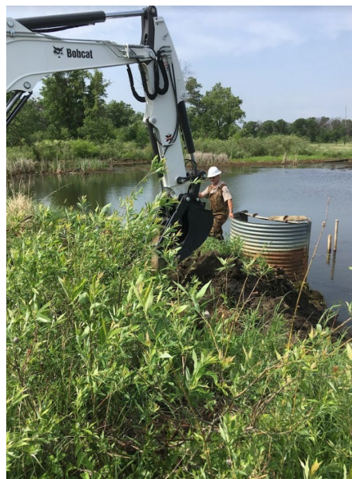
Active management of land and water resources supports conservation and wildlife dependent recreation. At Rice Lake NWR (MN), installation of a beaver deterrent helps maintain appropriate water levels and prevents flooding. Credit: USFWS
