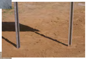
Fracturing Sign Support
